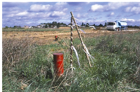
Marking of a point that will be the center of the synchrotron ring
